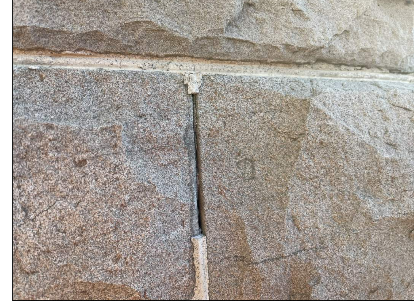
8 FAILED MORTAR JOINT SCALE: NTS
