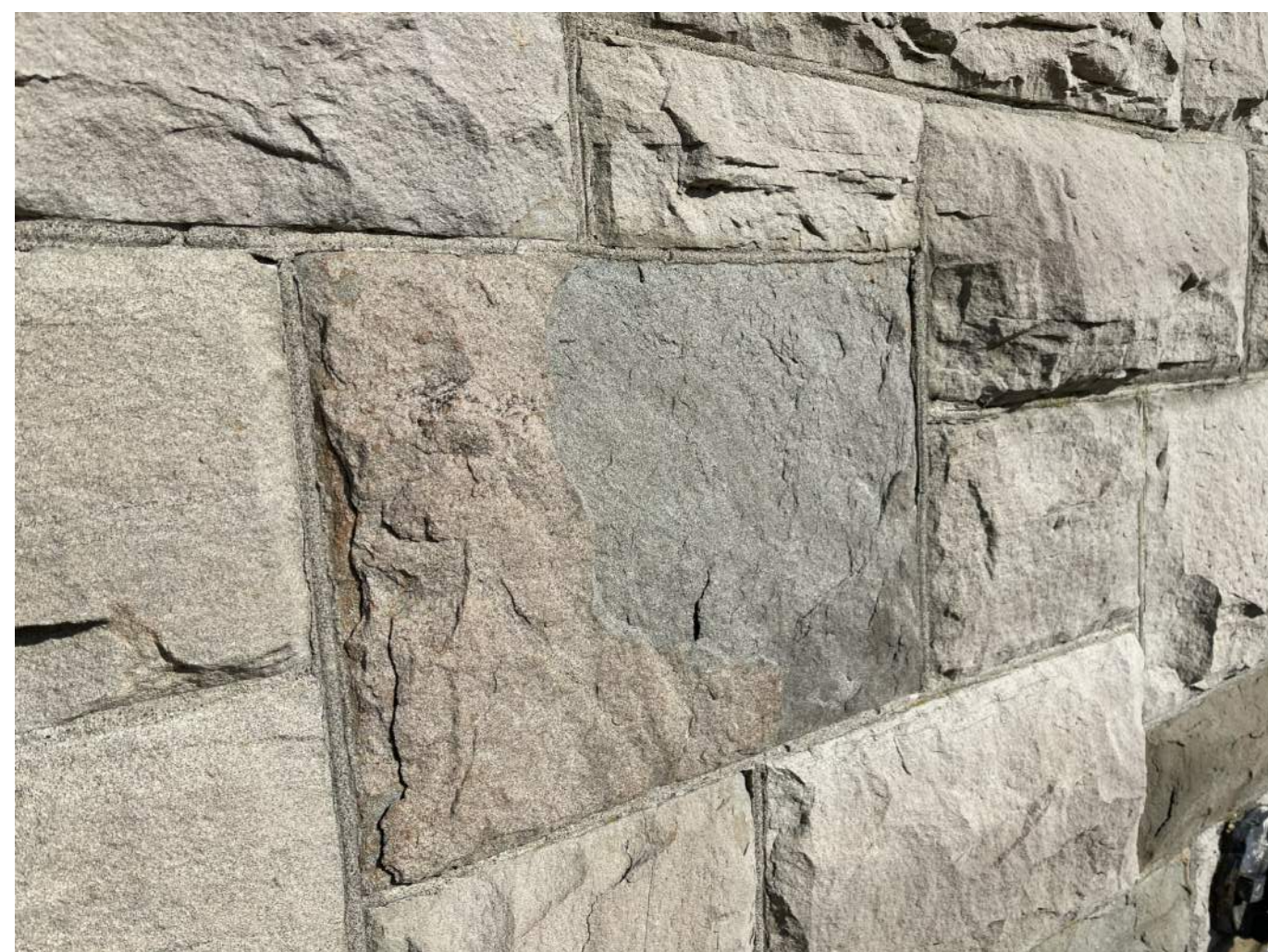
9 FAILED FACE AT FIELD STONE SCALE: NTS
