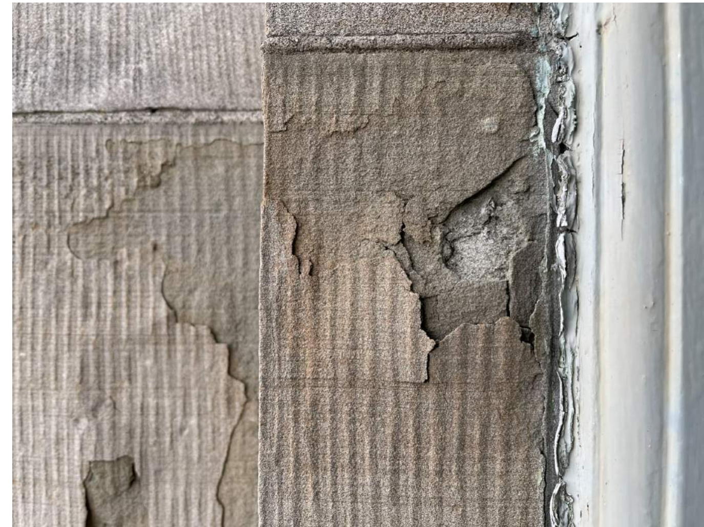
6 SPALLING AT WINDOW JAMB SCALE: NTS
