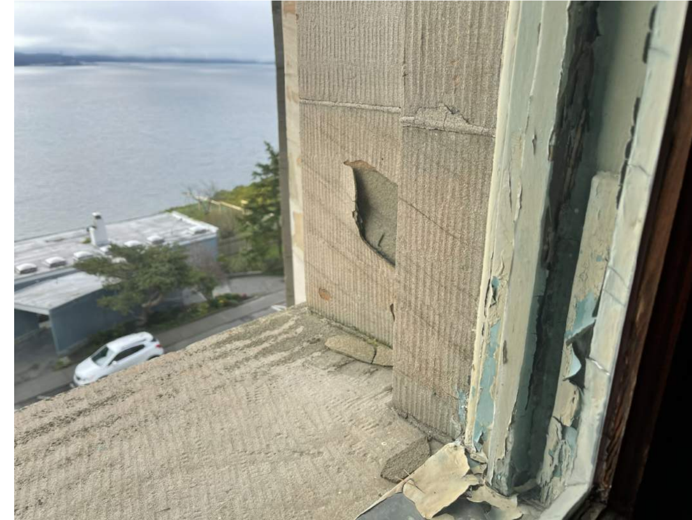
7 SPALLING AT WINDOW JAMB SCALE: NTS
