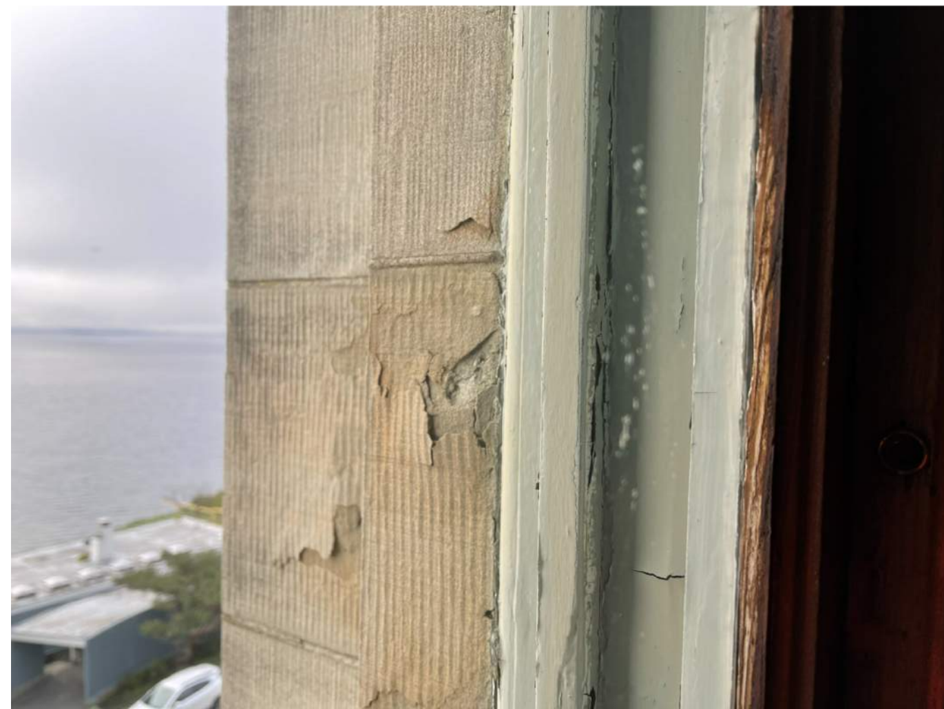
5 SPALLING AT WINDOW JAMB SCALE: NTS
