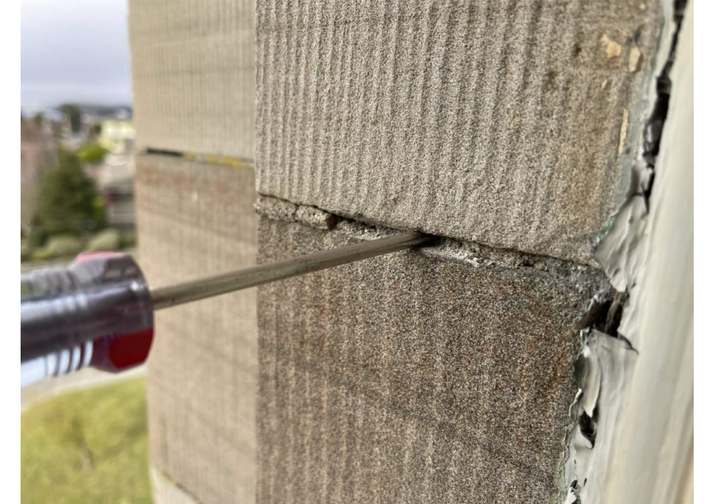
8 FAILED MORTAR JOINT SCALE: NTS
