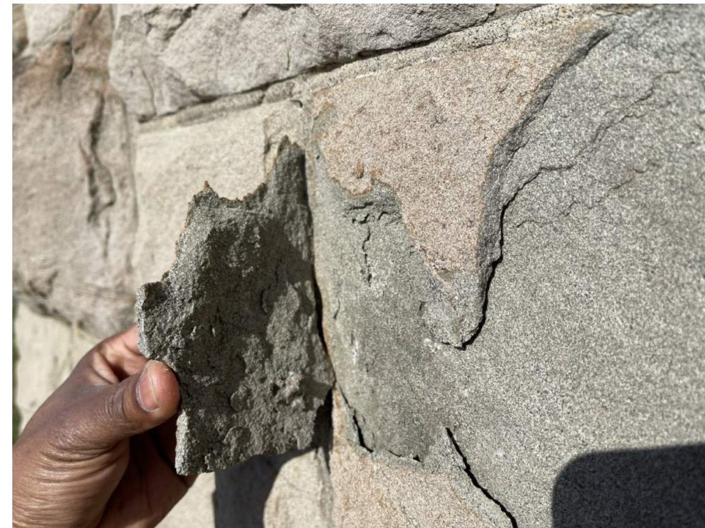
10 FAILING FACE AT FIELD STONE SCALE: NTS
