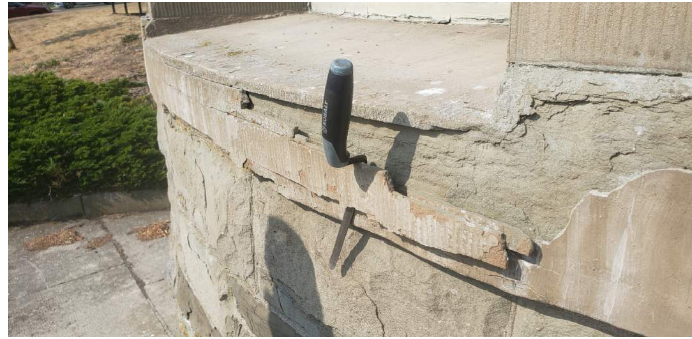
1 SPALLING AT SILL FACE SCALE: NTS
