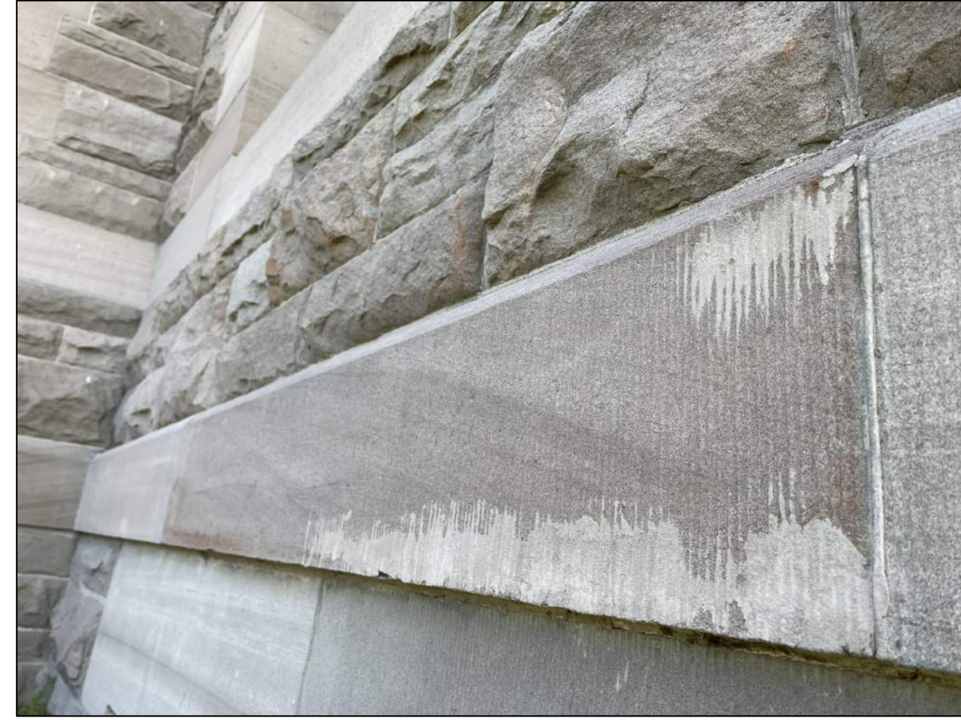
2 PREVIOUS PATCH AT WATER TABLE SCALE: NTS
