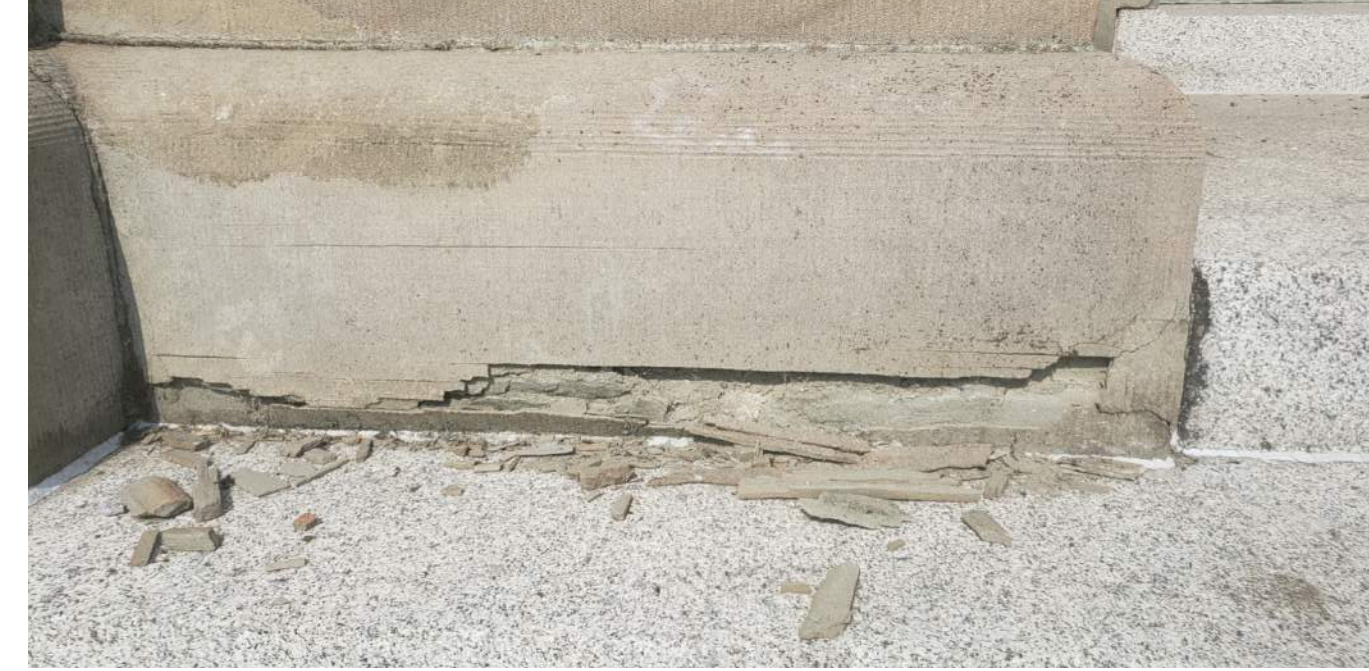
3 SPALLING AT FRONT ENTRY SCALE: NTS
