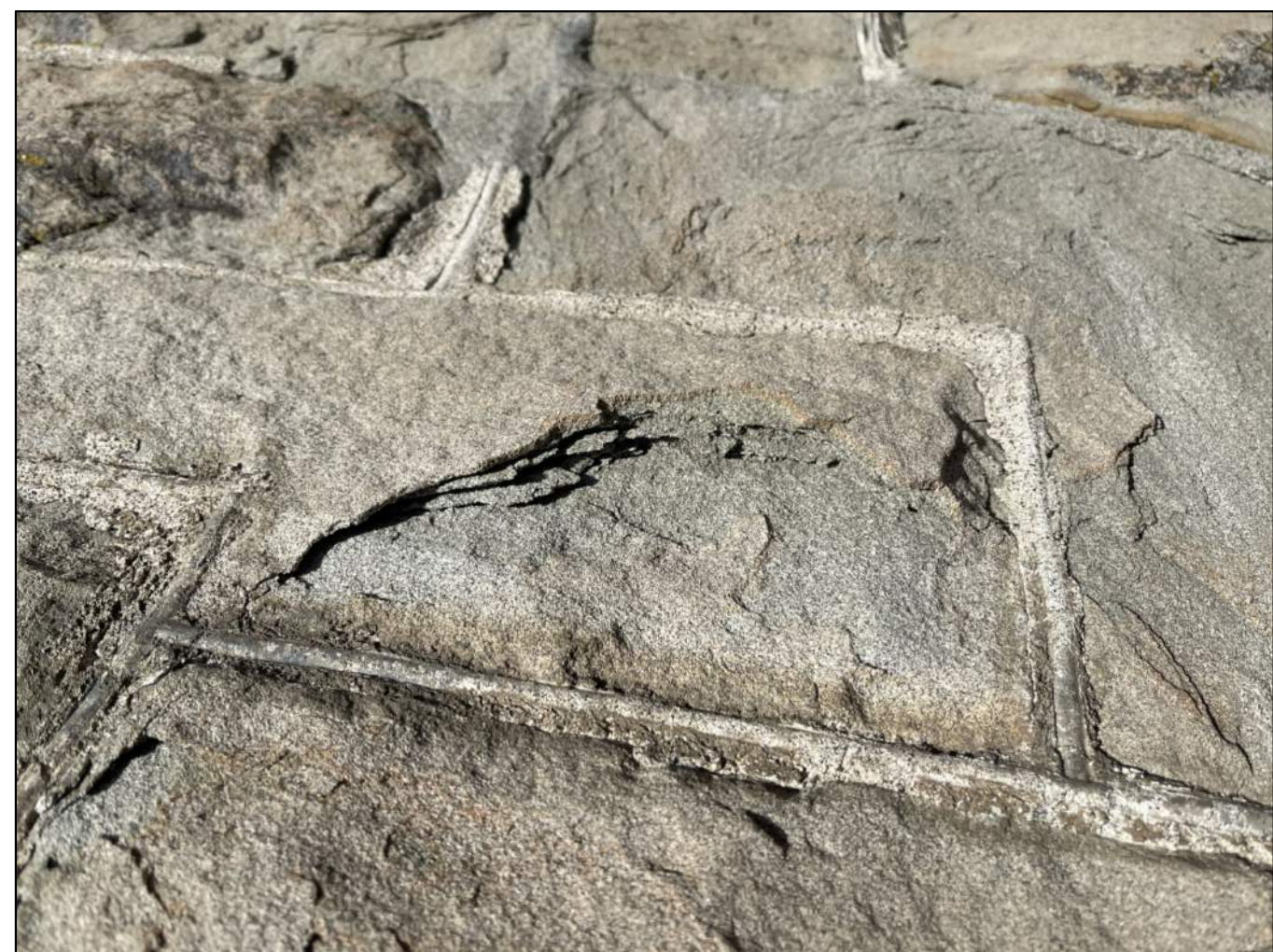
9 FAILED FACE AT FIELD STONE SCALE: NTS
