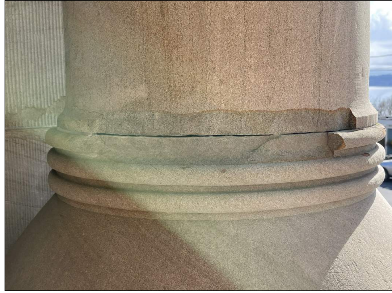
5 CRUMBLING COLUMN PROFILE SCALE: NTS
