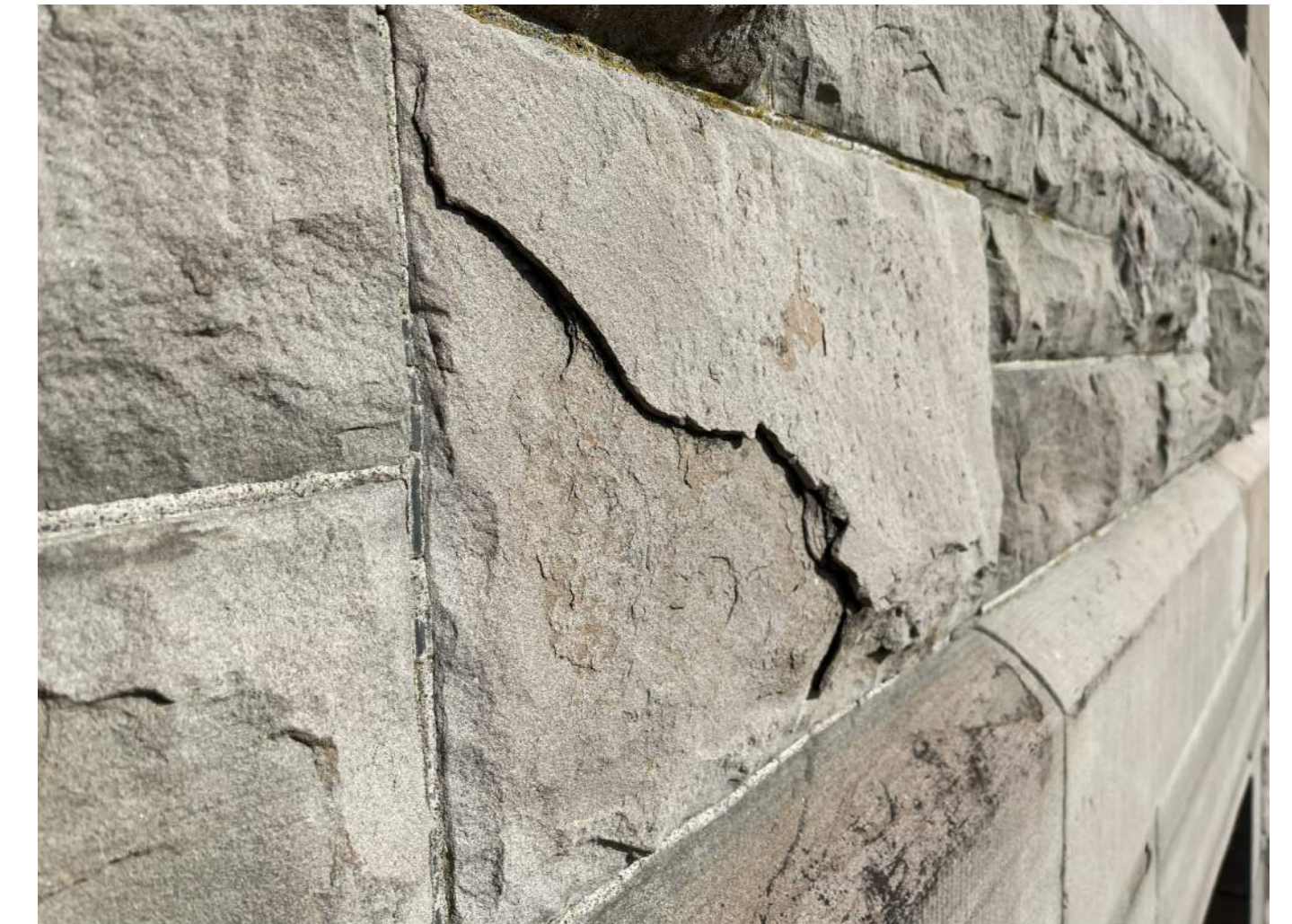
12 FAILING FACE AT FIELD STONE SCALE: NTS
