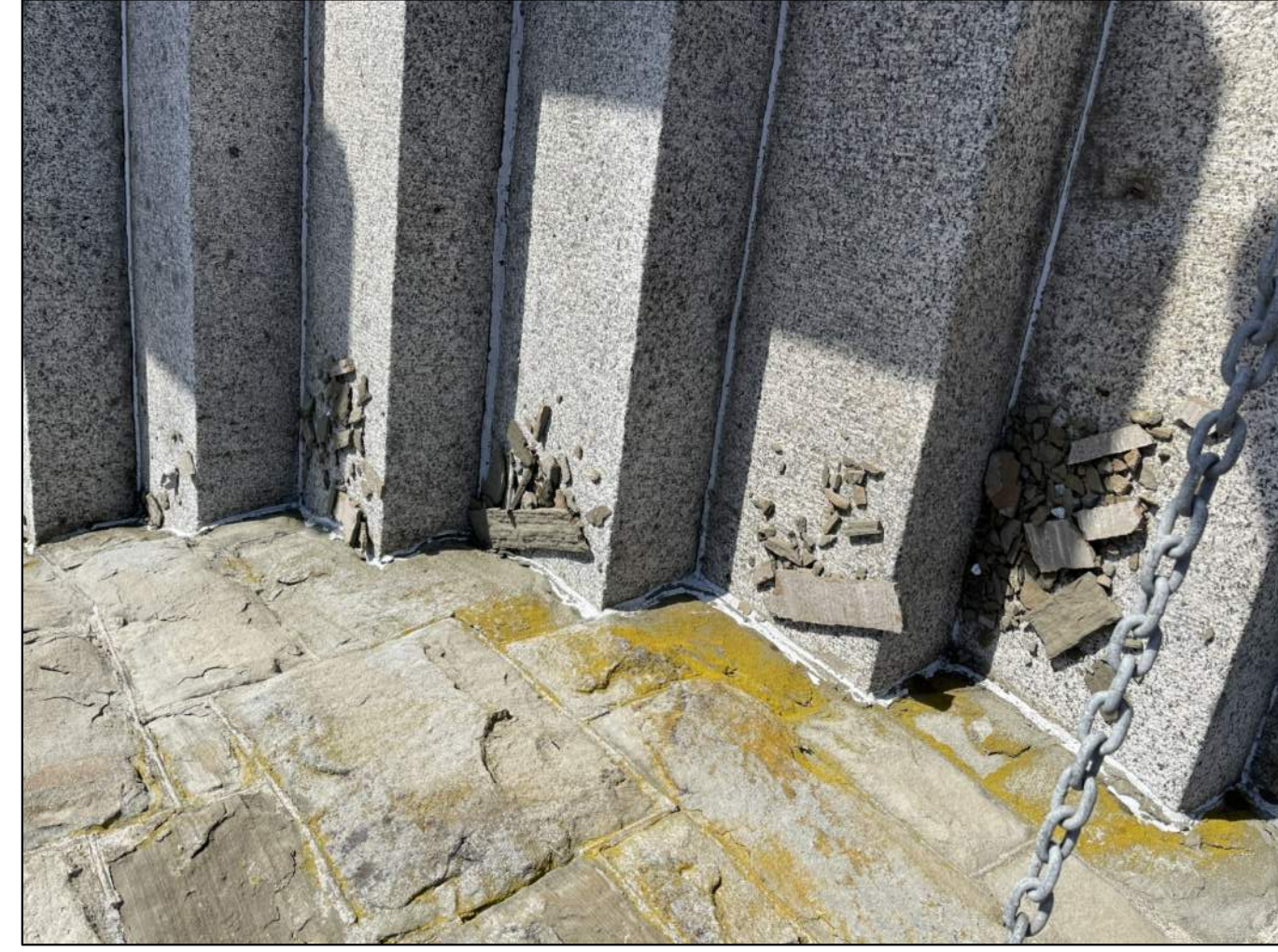
6 FALLEN STONE FRAGMENTS ON STAIRS SCALE: NTS
