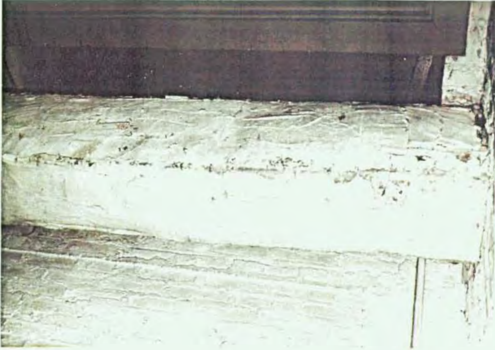
View of Damaged Asbestos Insulation on an Exposed Duct in the Mechanical Room.
