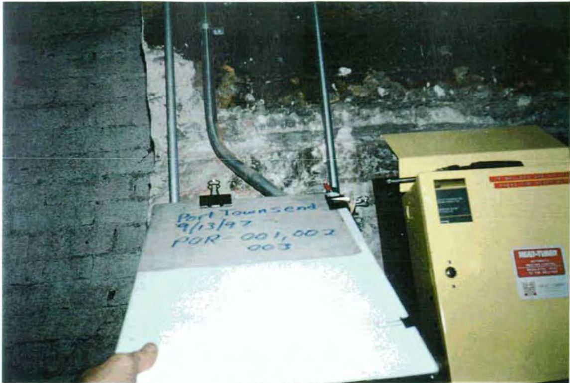
Debris on Brick Ledges Sample Numbers: 001, 002, 003 Homogeneous Material Photograph
