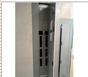
20 PHOTOGRAPH - INSIDE PANEL G
