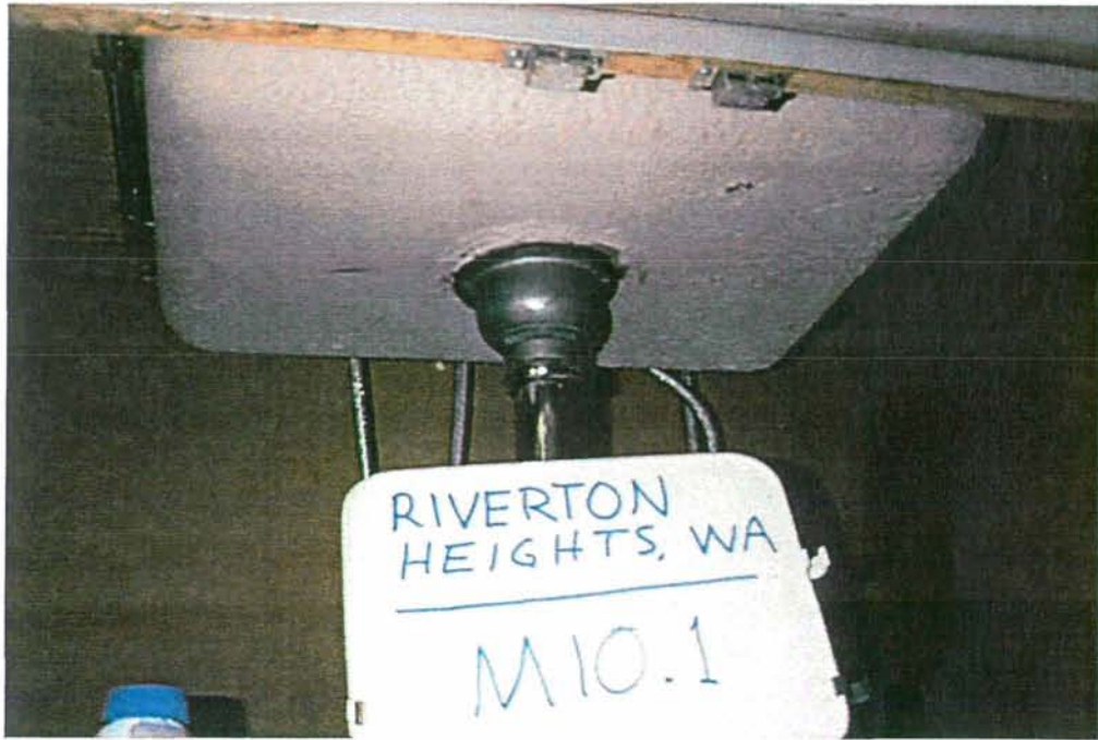
PHOTO #5 - UNDERCOATING ON SINK (M10.1)
