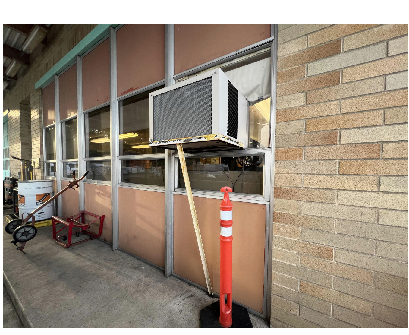
Detail: Fac. | Ch. | Sect. | Para. | Detail CAD File: Scale: USPS SDL Issued: Last Revised:
