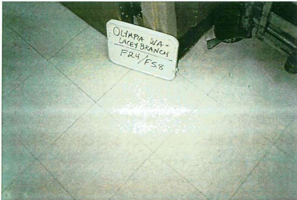
PHOTO #6 - MASTIC UNDER 12"x12" BEIGE WITH LINES FLOOR TILE (F5.8)
