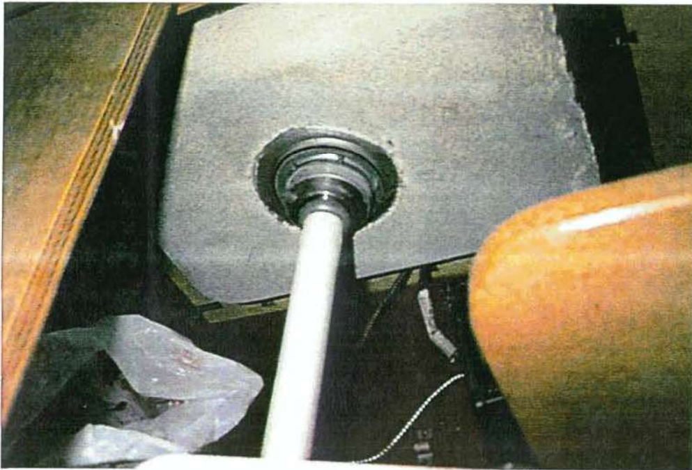
PHOTO #8 - SINK UNDER COATING (M10.1)
