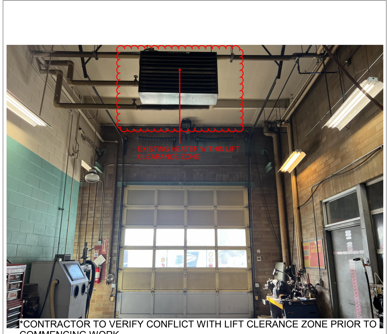
13 POTENTIAL OBSTRUCTION AT WASH BAY CONTRACTOR TO VERIFY CONFLICT WITH LIFT CLEARANCE ZONE PRIOR TO COMMENCING WORK
